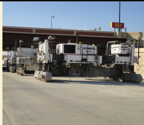
(Pictured: Crews recently paved the westbound SH 114 mainlanes from Main Street to William D. Tate Avenue.)
