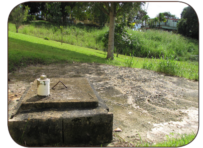
Keep septic tanks sealed.
